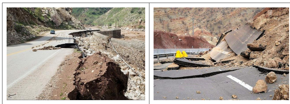
Fig. 7: Images of landslides in the study area
